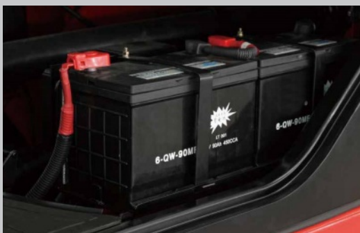
The battery is located above the fuel tank.
